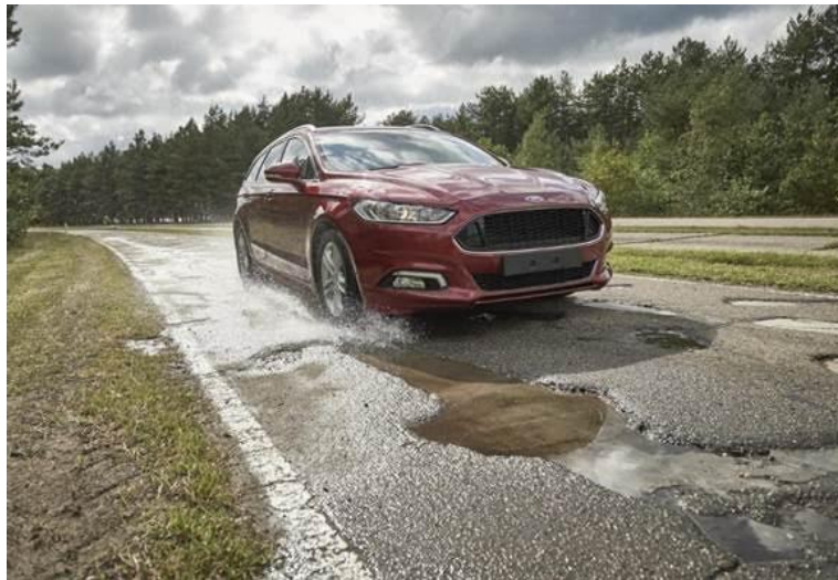
Figure 1.1. Poor pavement condition may contribute to driver distraction, substandard vehicle operation and accidents ( http://www.carprousa.com/bumpy-commute-try-driving-on-fords-pothole-road )
