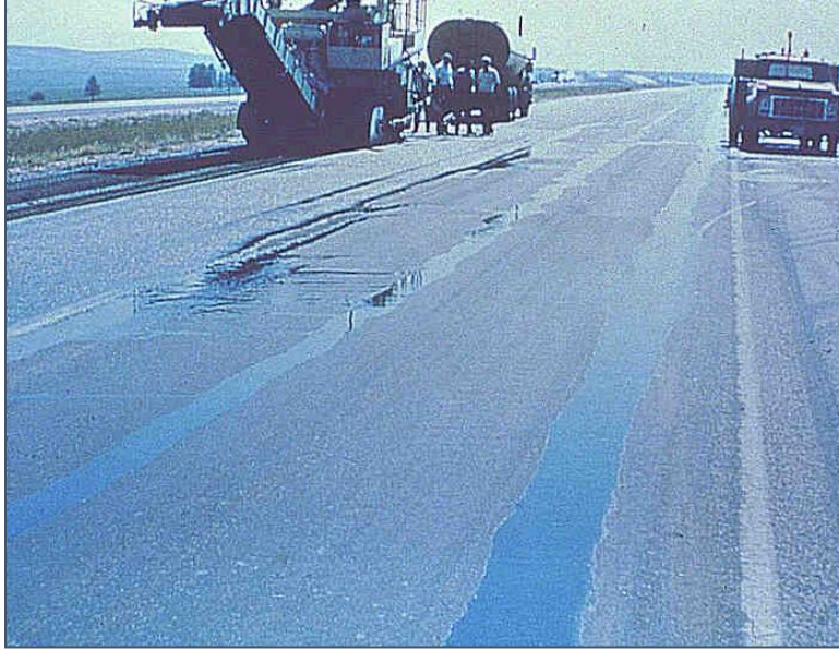
Figure 2.3. Example of pavement rutting with water accumulation (Miller and Bellinger 2003)
