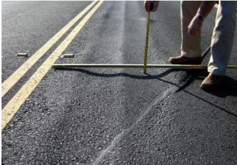
Figure 1.2. Example of pavement rutting ( http://www.qespavements.com/node/113 )
